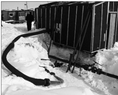
(← Fig. 6.6) The onshore Pump Station
