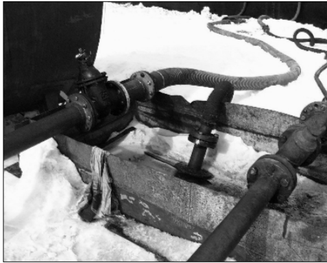
(← Fig. 6.3) Hoses connected to the hand driven valves of the pipeline
