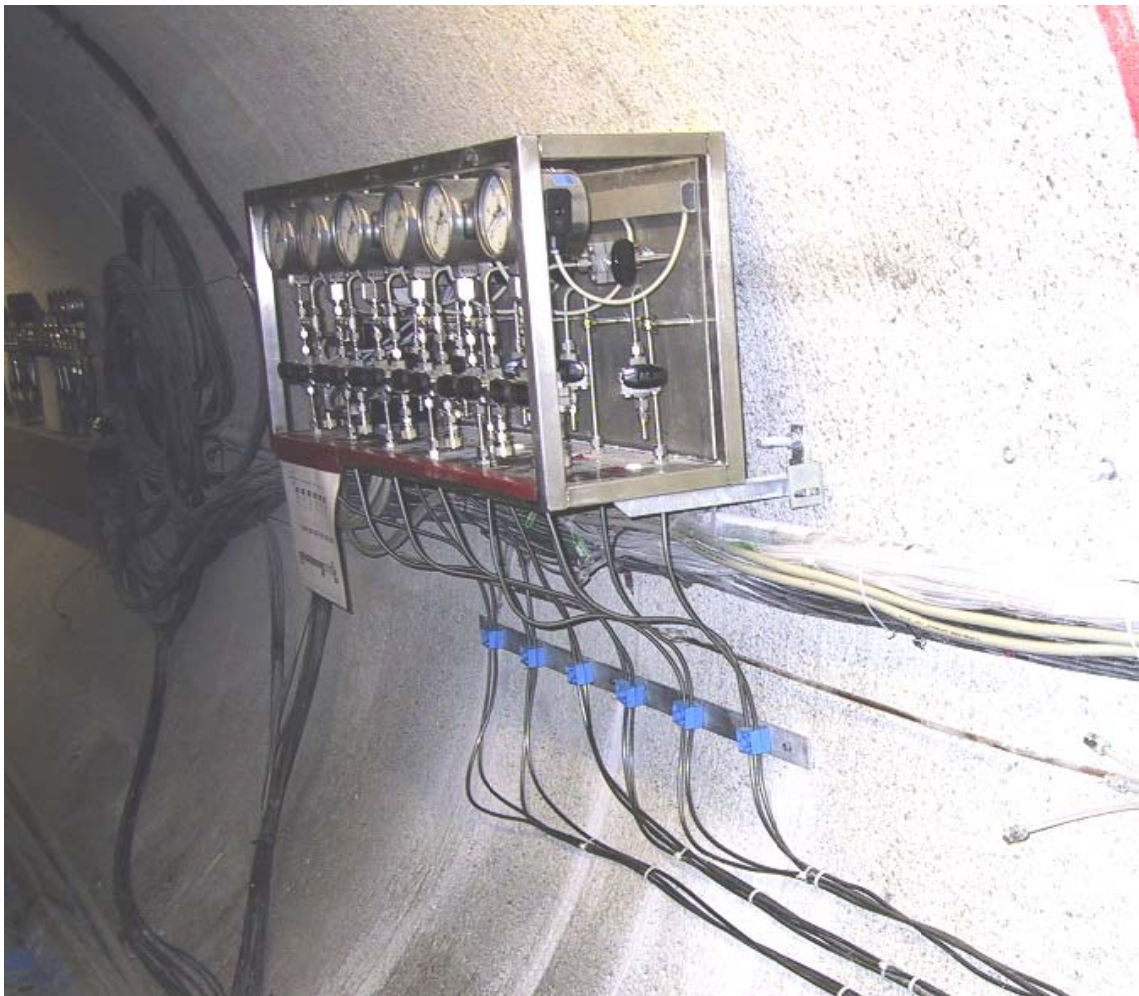
Fig. 2.18 Valve panel with the pressure gauges, flow meters and capillaries from the draining pipes
