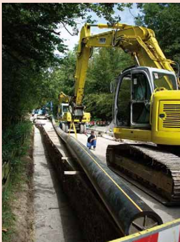
Figure 14: Micro biogas pipeline: In this system, the biogas is transported to the heat sink without upgrade and feed-in into the natural gas pipeline. Thus, the total efficiency is increased without energy intensive upgrading
