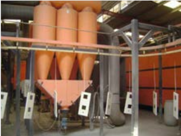
Conveyor belt for powder coating (Source: Copyright by UNIDO)
