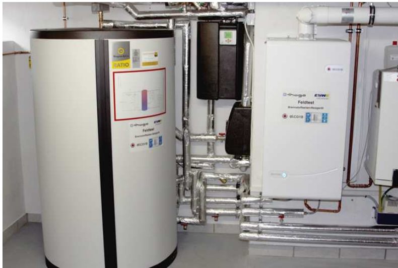
Installation in Wiesbaden
