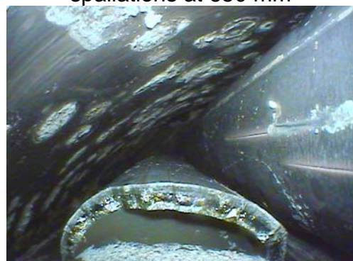
rod 16 break and rod 27 cracks at 900 mm
