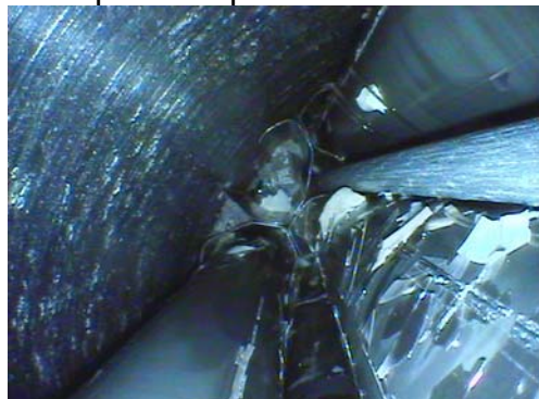
spallations at rod 16 at 500 mm
