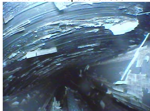
spallations at 650 mm
