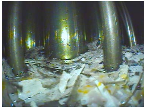
debris on bottom of separator
