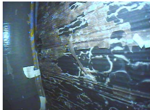
spallations at shroud at 400 mm
