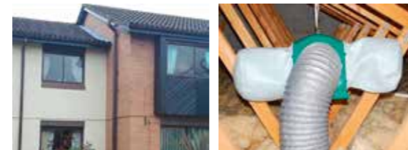
Figure 2 externally located sump system (left), whole house ventilation system (right)
