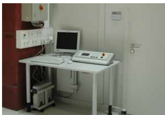
Fig. 2 Control unit of the Isovolt X-ray tube in front of the laboratory.
