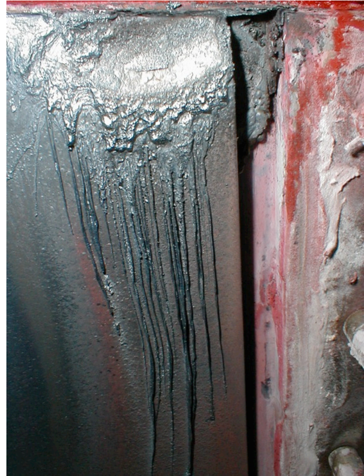
Melted carbon steel sidewalls. Slot for panel shown.
