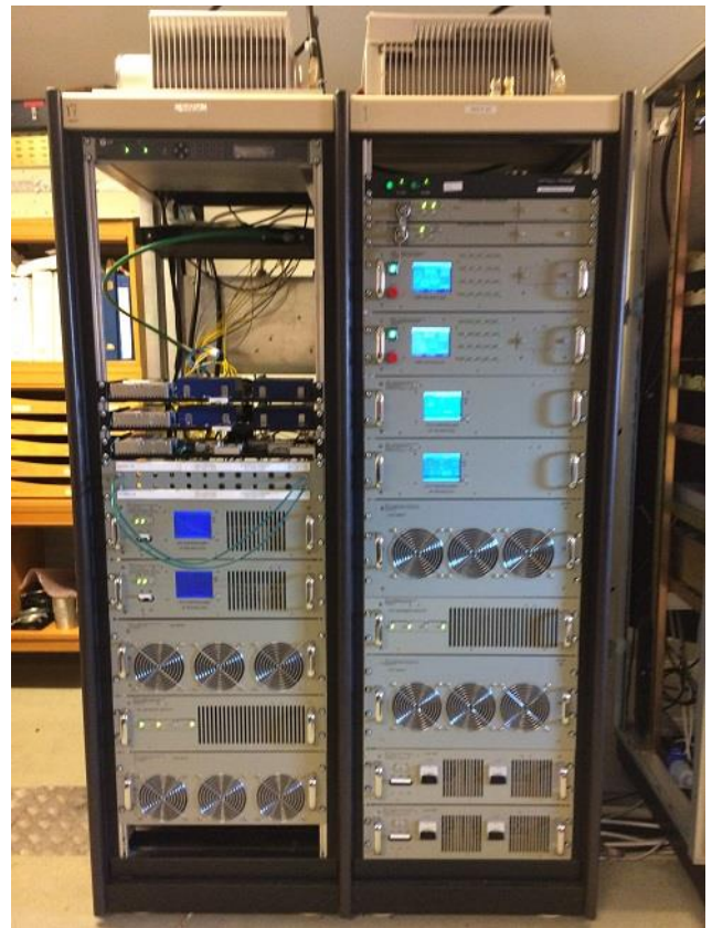
Figure 5 Transmitter rack at transmitter site
