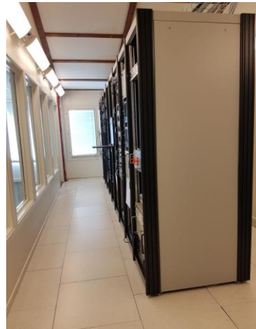
Figure 5. TMR; New data floor. Nine new telemetry racks, 44RU.
