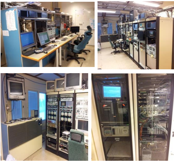
Figure 3. Old TM-station. Equipment in different racks.
