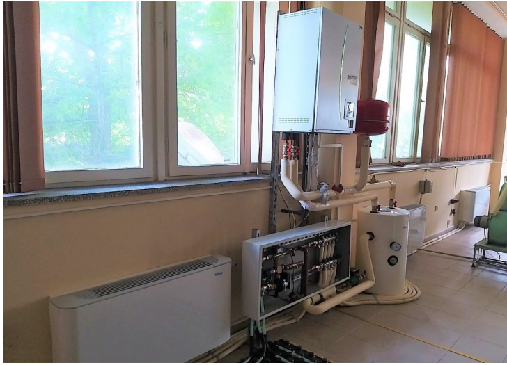
Fig. 2. General view of the AHP system.
