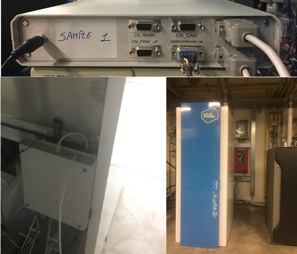
Figure 2. MDLT mounted on the EnGen-2500 system from SOLIDpower: top: MDLT; bottom left: location of the MDLT at the back of the SOFC EnGen-2500 system; bottom right: front side of the EnGen 2500 installed in its testing location
