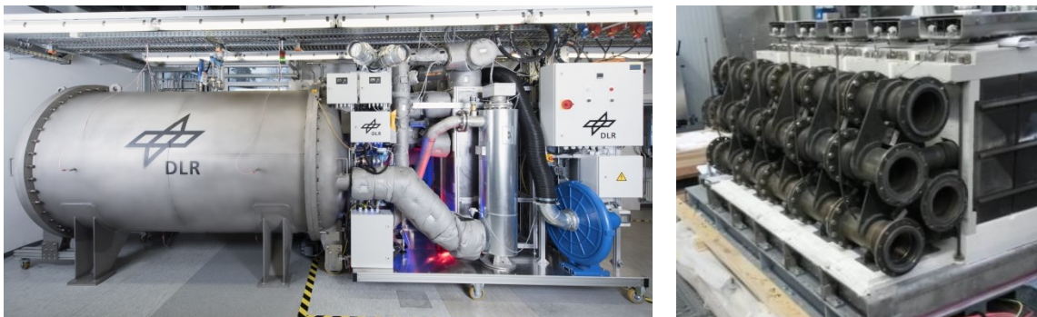
Figure 1: The pressurized 30 kW SOFC system with fuel gas recirculation at reaction temperature. It contains the shown 30 kW SOFC reactor.
