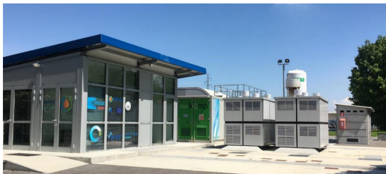
Figure 3. SOFC modules and the DEMOSOFC site.
