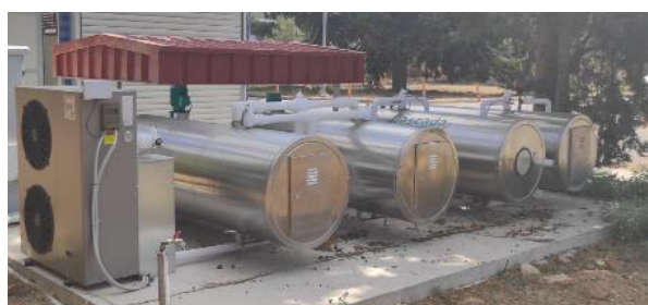
Fig. 6. Hot and cold water tanks and pumps for the compressor operation
